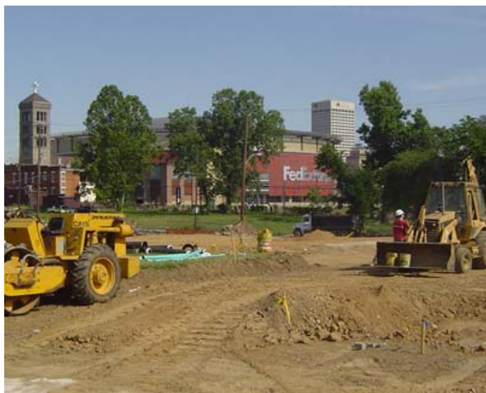
View of the FedEx Forum (background) from the site of the new Streets Center
