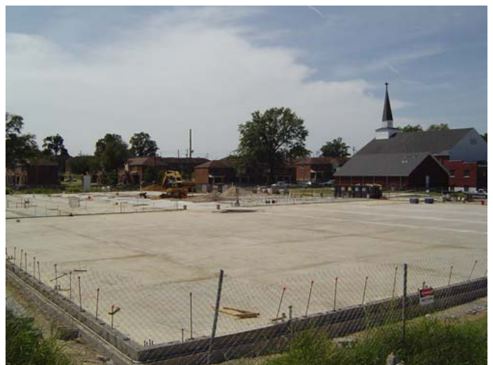
On September 23rd, the concrete pad was completed and our new 35,000 square foot facility began to take shape.
