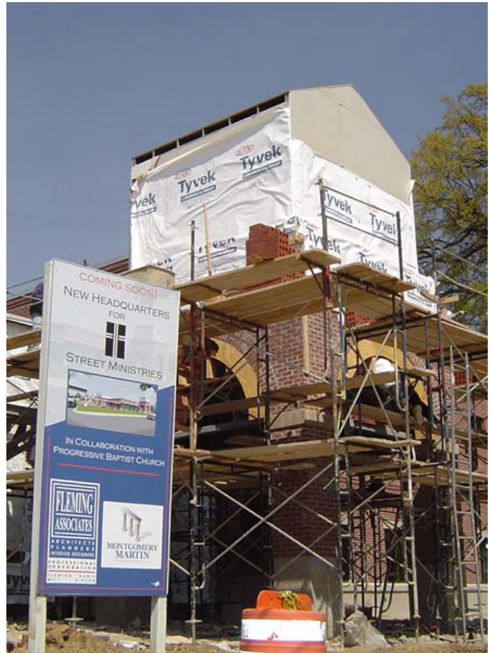
As brickwork along the main entrance facing Foote Homes nears completion, the rendering becomes reality.
